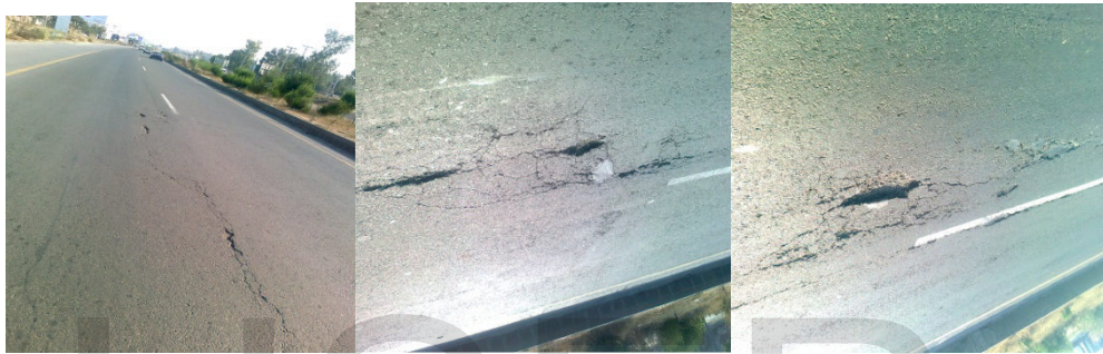
Low severity pot holes at KM 1542+950NBC
