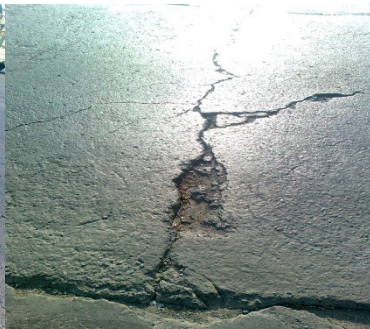
High severity reflection cracks at KM 1493+350 NBC
