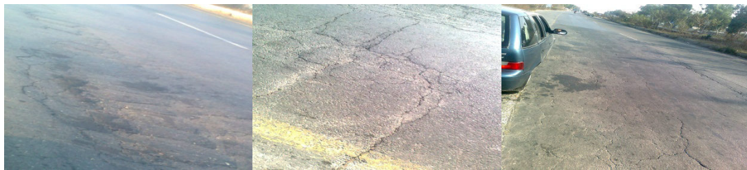
Low severity cracks At KM 1394+100 NBC
