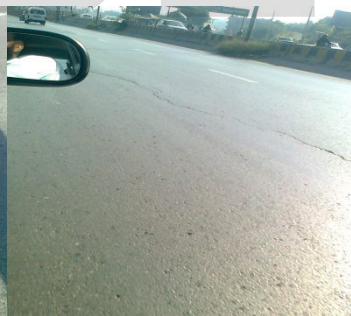
High severity cracks at KM 1528+400 SBC
