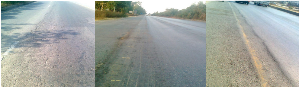
Low severity rutting At KM 1494+670 NBC
