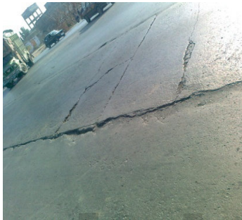
High severity reflection cracks At KM 1503+200 SBC
