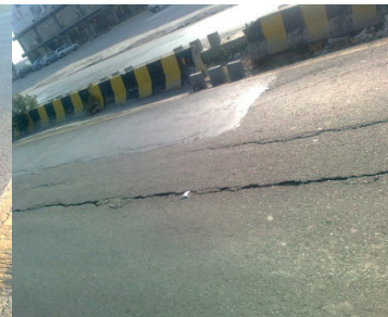
High severity patch at KM 1543+175 NBC
