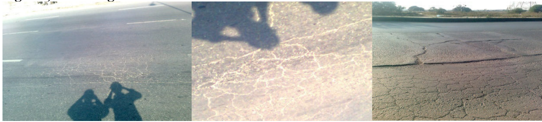
Low severity cracks at KM 1529+800 SBC
