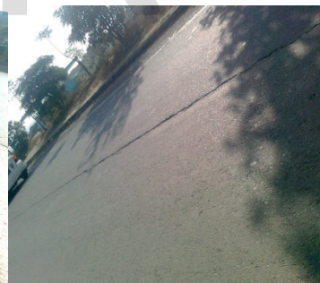
High severity cracks at KM 1517+900 NBC
