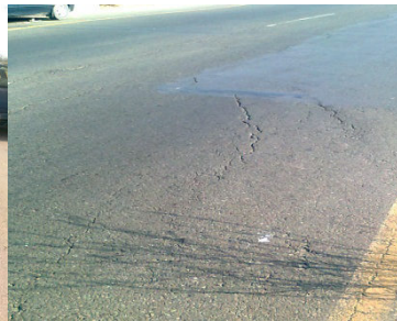
High severity patch at KM 1537+423 NBC
