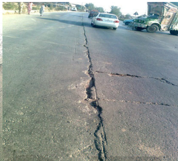
High severity reflection cracks at KM 1503+275 SBC
