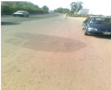
Low severity patch At KM 1512+221 NBC
